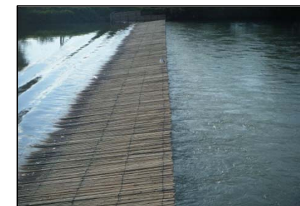
The reason for the gaps in the weir could have been caused by the garbage, e.g. fallen leaves, small pieces of trunks and stones in the water and a combination with water pressure.
